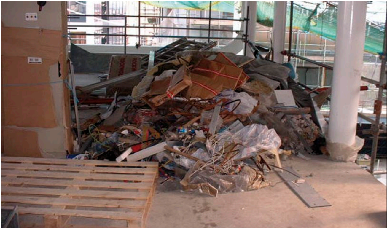
Figure 6 Most construction rubbish can burn. Make sure that it is swept up and removed from the site as soon as possible
